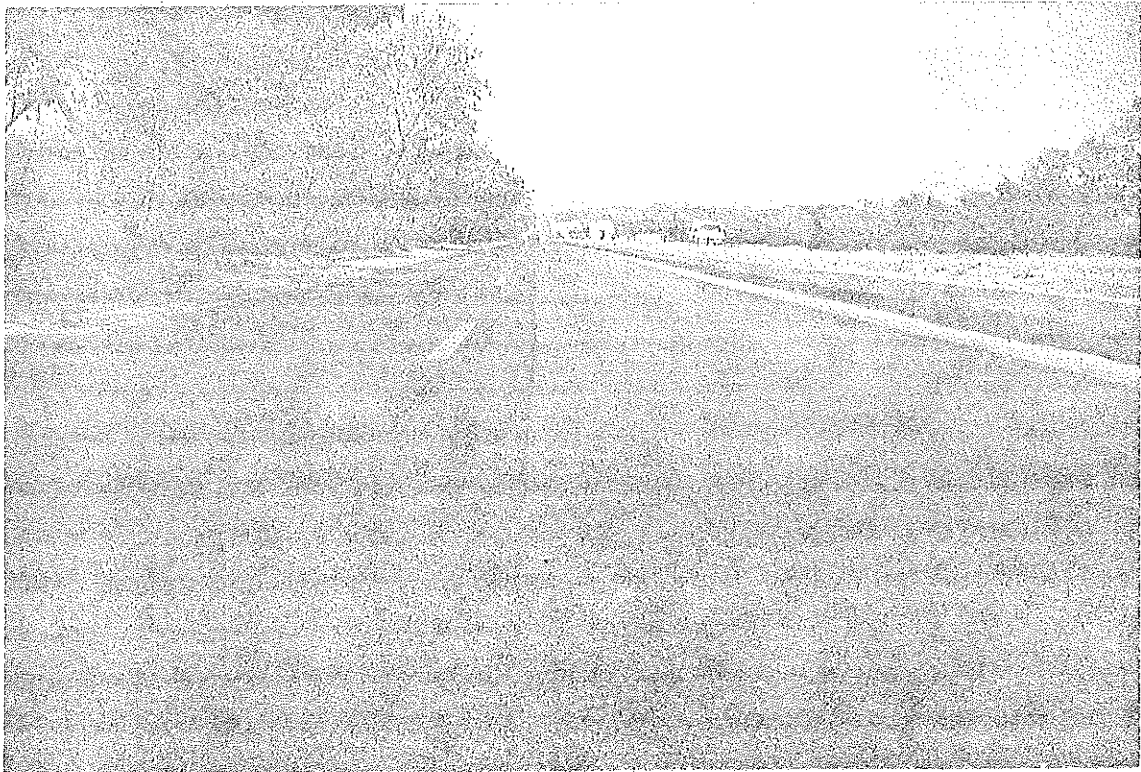
Plate 7.1(a) Completely milled outer lane of the old highway, exposing the texture to weathering. Polished surface of 2nd lane is also detectable.
